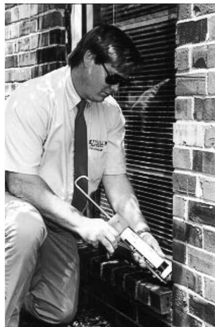
Figure 3. Sealing cracks and exterior openings provides long-term relief against pest entry.
