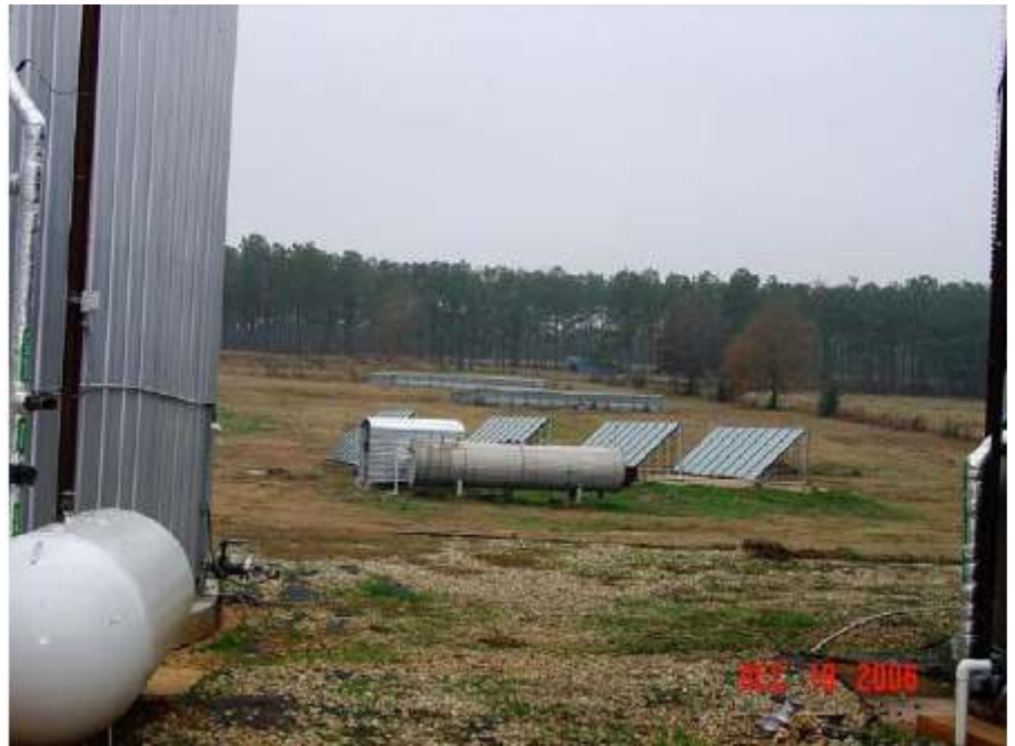
Photo shows the setup for heating the well water and burning the sawdust
