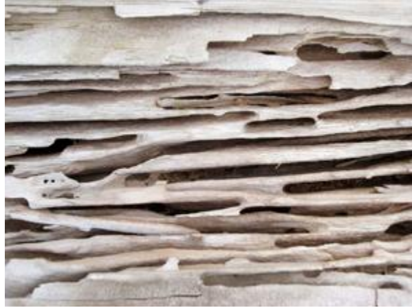
Clean carpenter ant galleries in wood (photo: mcinroybasementsystems.com)
