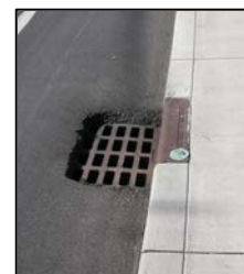
Existing hazardous drainage grate
