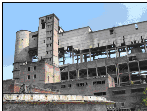
Figure 2. Defunct mercury processing plant at Nikitovka Mines, Gorlovka, Ukraine, operated from 1968 to 1991 (2005 photo).
