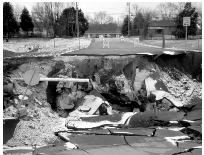
One of the hidden karst hazards: this highway near Bowling Green caved in as a result of sudden cover collapse.
