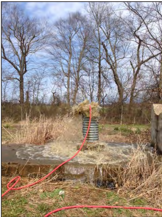
Figure 6. The air-lift method (using compressed air to surge the well water to clean out the well-casing screen) was used to redevelop the USGS Climate Response Network well in Graves County. A USGS video describing this procedure can be seen at www.usgs.gov/center-news/usgs-groundwater-monitoring-well-redevelopment-using-air-lift-method .
