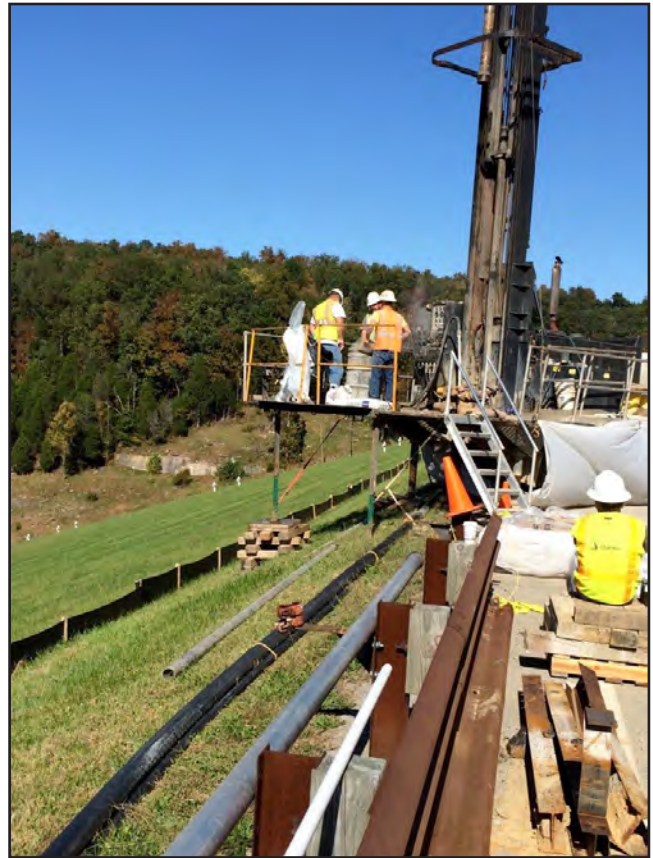
Figure 10. Contractors for the U.S. Army Corps of Engineers install vibrating-wire transducers on the downstream side of the Rough River Dam. The USGS monitors the transducers in cooperation with the Corps.
