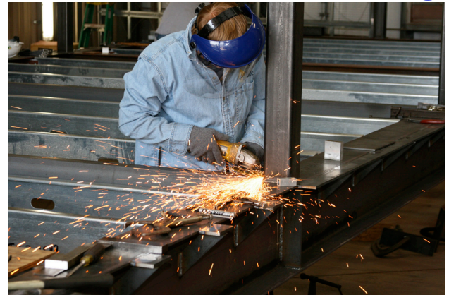
Ross Graham, a UK College of Design student works on the s.ky blue solar house structural frame
