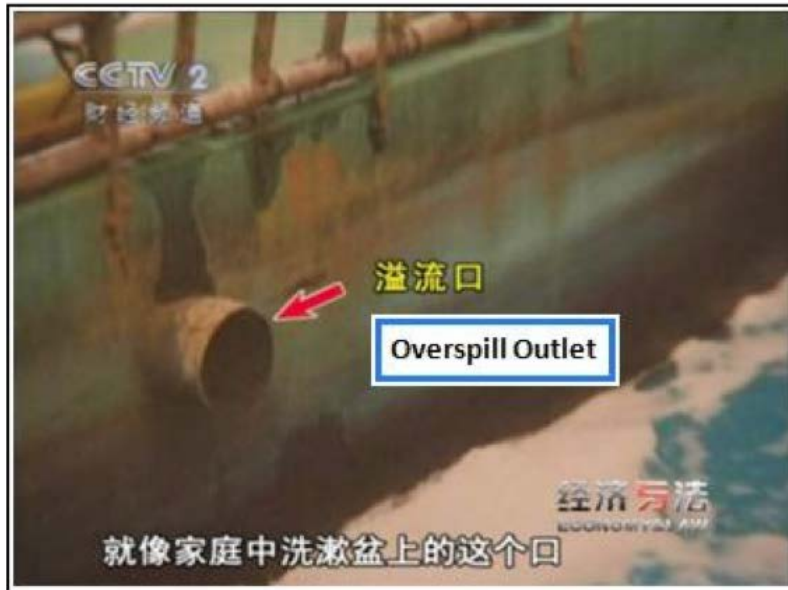
Figure 3: Overspill outlet adjusted over the pool
