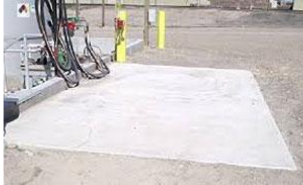
Impervious containment pad
