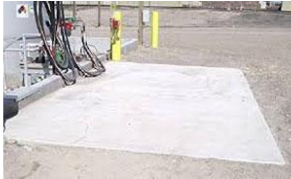
Impervious containment pad
