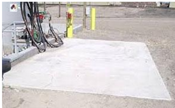
Impervious containment pad
