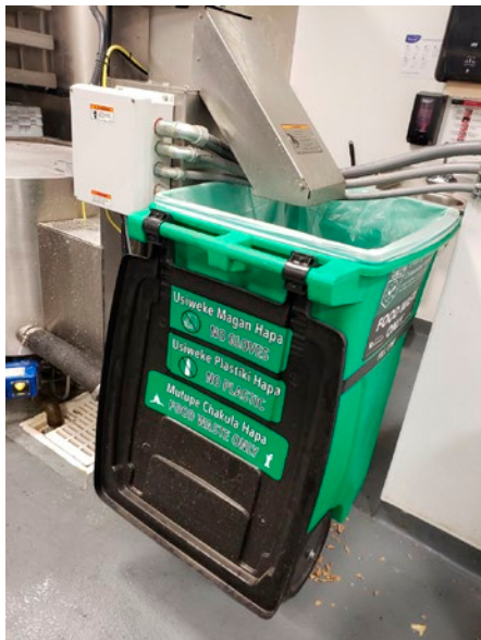
Food waste is sent through a pulper at each dining facility.
