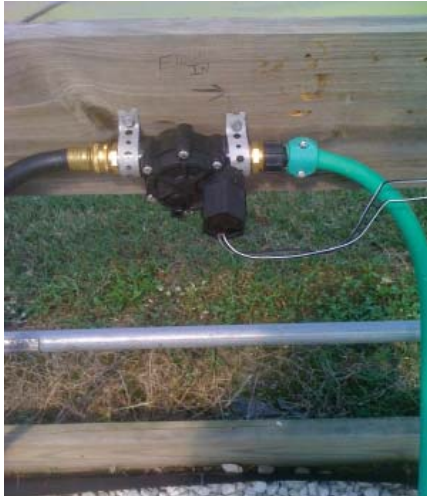
Hose from hydrant into solenoid and out to mist system.
